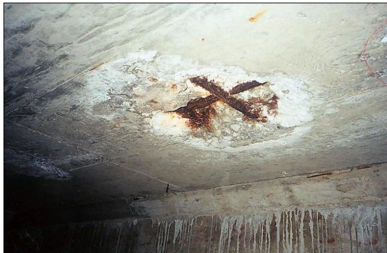
Figure 2.3.3.2-1: Localized Spall with Exposed/Corroding Rebar on the Deck Underside of a Post-Tensioned Box Girder.
