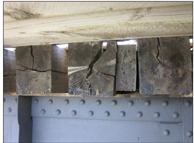
Figure 2.3.5.1-3: Timber Deck (Railroad Ties) – Condition State 3.
