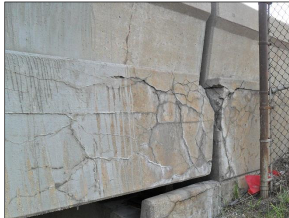
Figure 2.3.2.1-4: Typical Reinforced Concrete Slab Distress.
