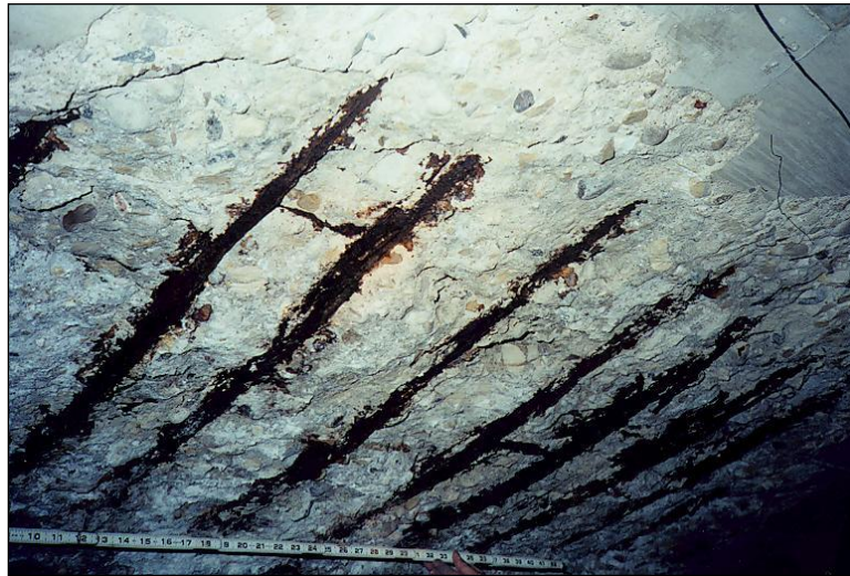
Figure 2.3.2.2-2: Reinforced Concrete Box Girder Top Flange/Deck Localized Rebar Corrosion and Bond Loss.
