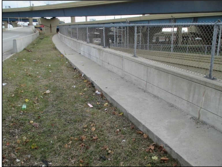
Figure 4.4.5-13: Drainage System Along Top of Retaining Wall. Note Vegetation Exhibits No Signs of Erosion or Settlement.
