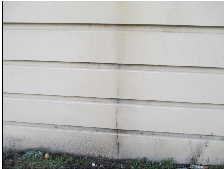
Figure 4.4.2-21: Vertical Crack Through Precast Concrete Panel.
