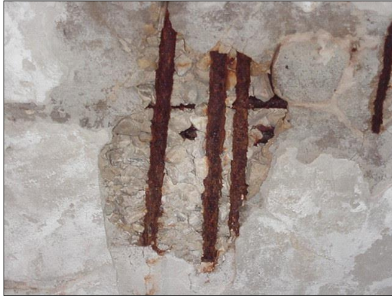
Figure 4.4.2-22: Concrete Spalling with Exposed Reinforcing Steel.
