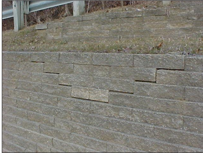
Figure 4.4.2-13: Poor Construction Methods Resulting in Block Separation.
