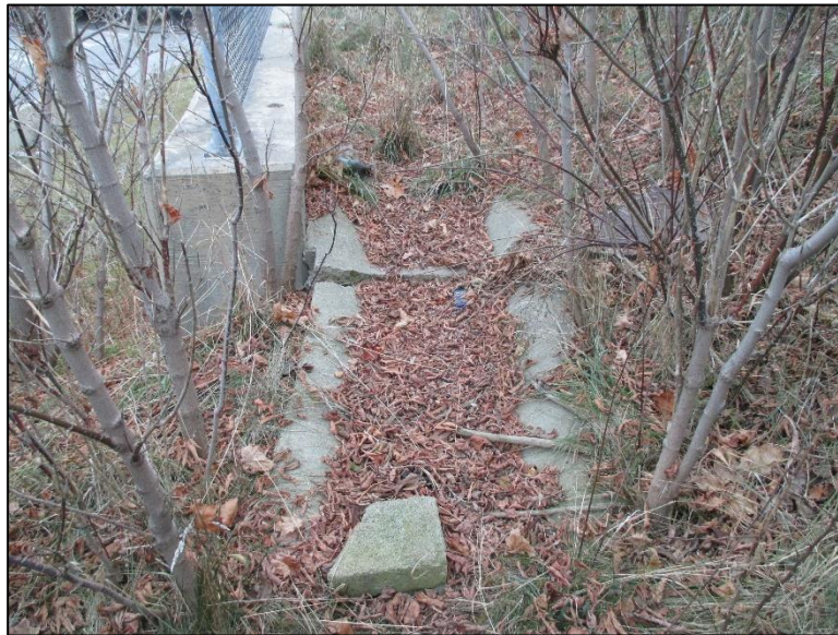
Figure 4.4.5-1: Concrete Flume at End of Wall. Condition State 2 (Fair) – No Erosion Evident, with wide crack.
