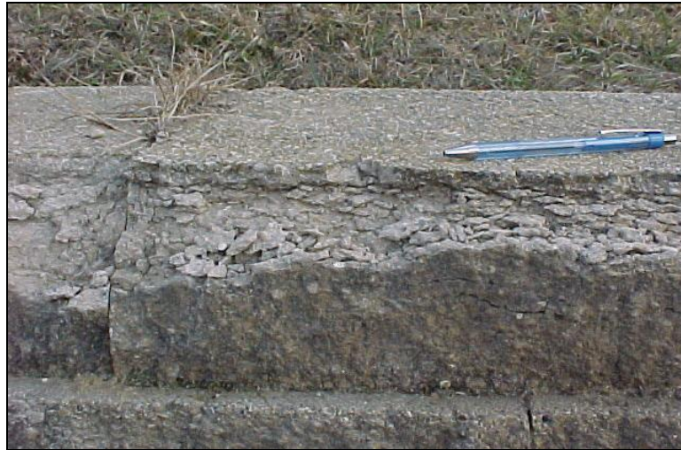
Figure 4.4.2-18: Freeze-Thaw Damage at a Corner.
