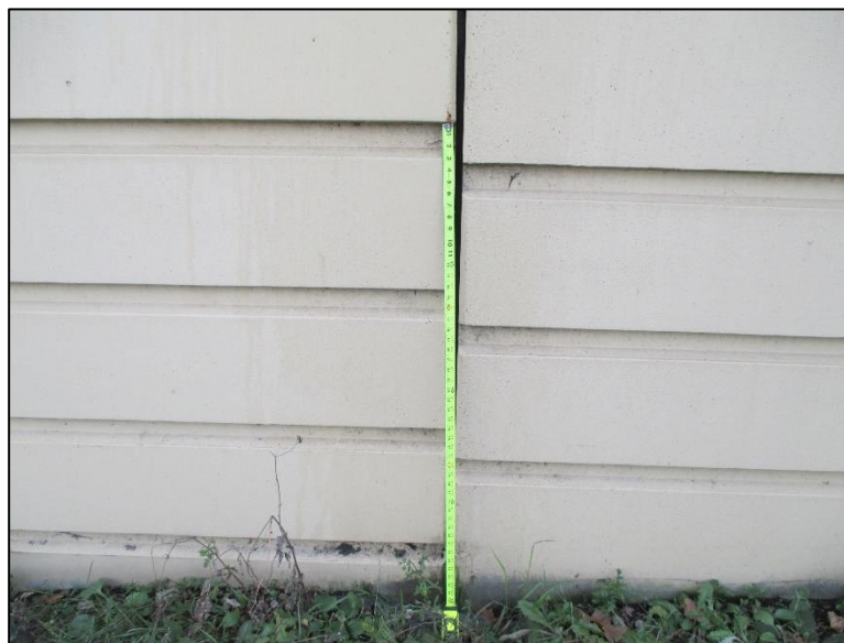
Figure 4.4.2-8: View of Differential Settlement between Precast Concrete Panels. Note Misalignment in Rustication.
