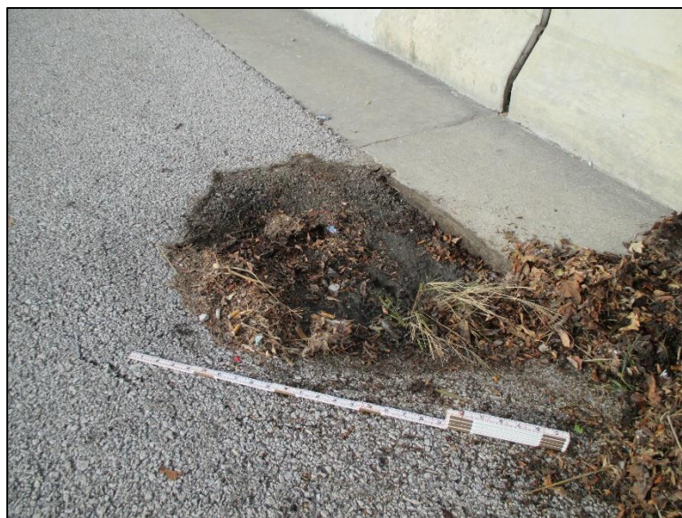
Figure 4.4.5-12: Pothole Due to Loss of Fill Within Shoulder Gutter Pan Along Top of Retaining Wall.
