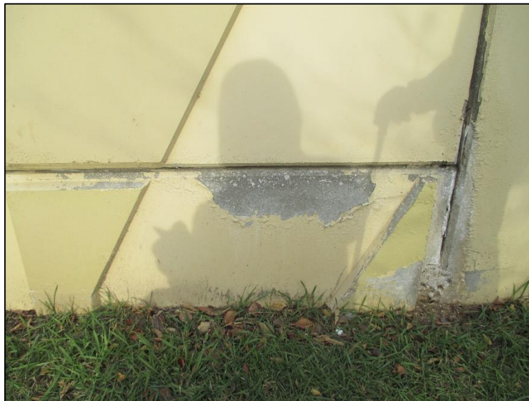
Figure 4.4.5-2: Failed Concrete Stain.
