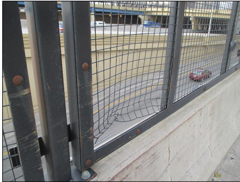
Figure 4.4.5-9: Assessment State 3 Protective Screening atop Bridge Rail. Note Chain-link Fence Deformation but Function Remains.
