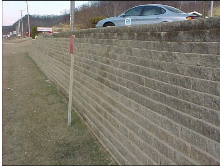
Figure 4.4.2-19: Typical Staining Evidenced by the Brown Discoloration of the Blocks.
