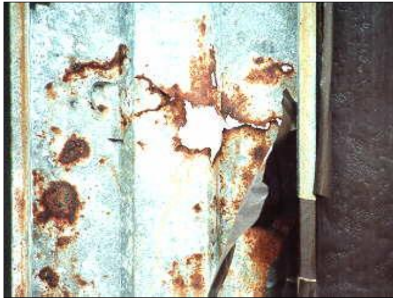
Figure 4.4.2-23: Severely Corroded Steel Sheeting Cantilever Wall.
