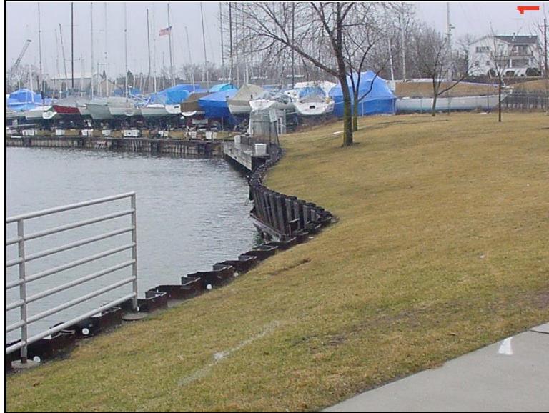
Figure 4.4.4-11: Tilted and Deformed Sheet pile Dockwall.
