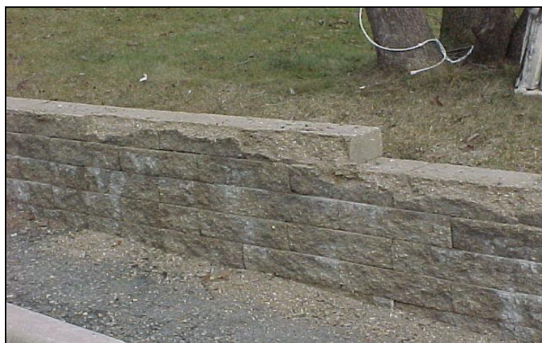
Figure 4.4.2-16: White Precipitate Formed due to Efflorescence.
