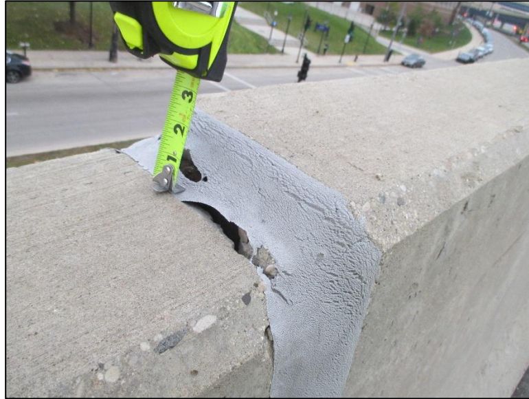
Figure 4.4.2-9: Settlement as Seen from Bridge Rail at Top of Wall. Note, Settlement was Reflected in Adjacent HMA Pavement.
