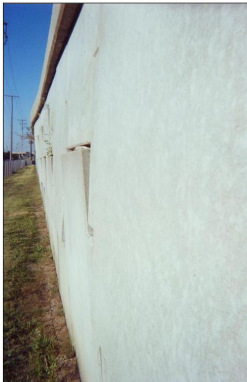
Figure 4.4.2-11: Lateral Movement of an Individual Panel of a MSE Wall.
