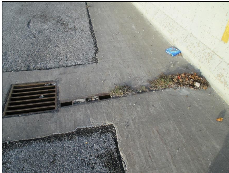
Figure 4.4.5-14: Drainage System Located along Top of Retaining Wall.
