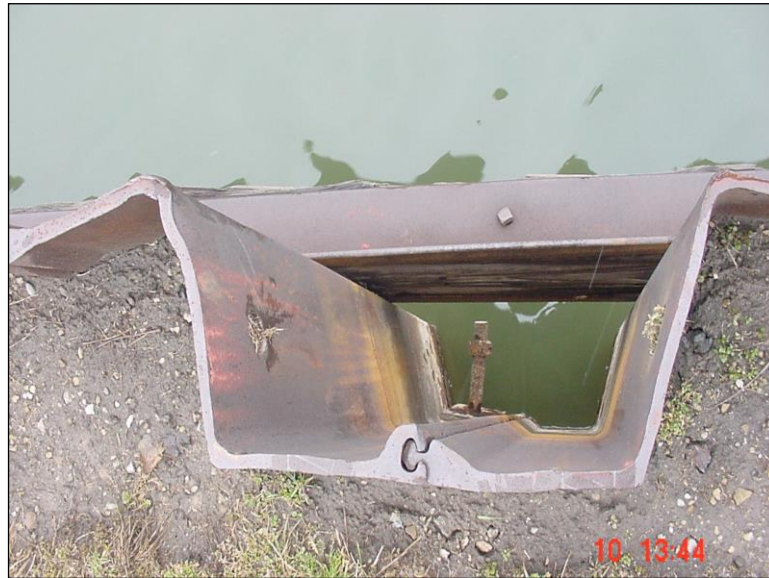
Figure 4.4.4-12: Failed Tie-rod Along a Sheet Pile Dockwall.
