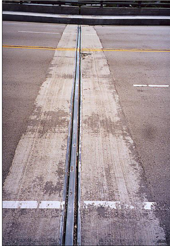
Figure 2.6.4.4-1 Modular Expansion Joint – Condition State 1
