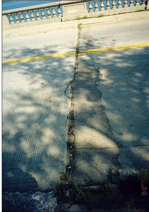
Figure 2.6.4.2-1 Poured Joint Seal – Condition State 3
