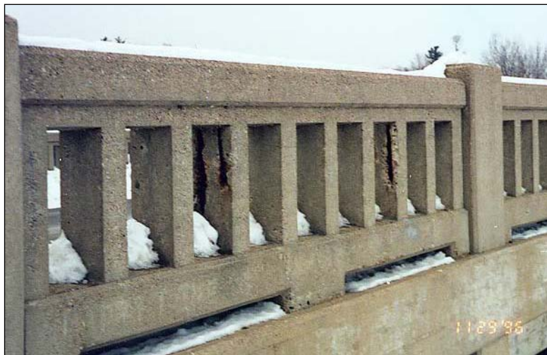
Figure 2.6.7.2-2 Concrete Bridge Rail – Most in Condition State 1 - Two Areas Condition State 3.
