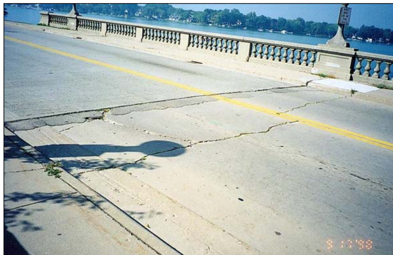
Figure 2.6.2.2-1 Concrete Approach with Wide Cracks – Condition State 3
