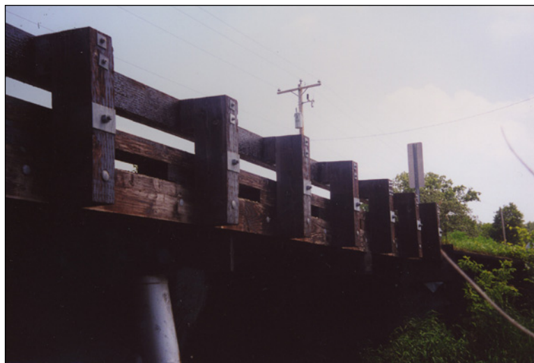
Figure 2.6.7.3-1 Timber Bridge Railing - Condition State 1
