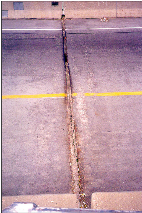
Figure 2.6.4.3-1: Compression Joint Seal Impacted with Debris and Pushed Down Into the Joint Opening (Far Lane)– Condition State 4.
