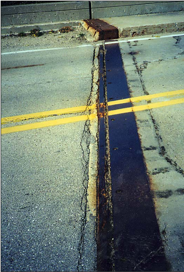
Figure 2.6.4.6-1: Sliding Plate Expansion Joint (Note Transverse Deck Crack on Left Side Suggesting a Failing Anchorage System) – Condition State 2.
