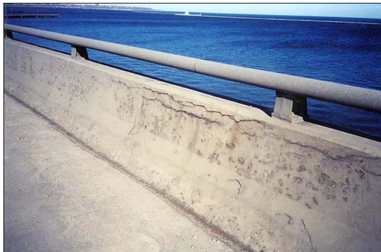
Figure 2.6.7.2-6 Concrete Railing with Decorative Rail Assessment – Condition State 3
