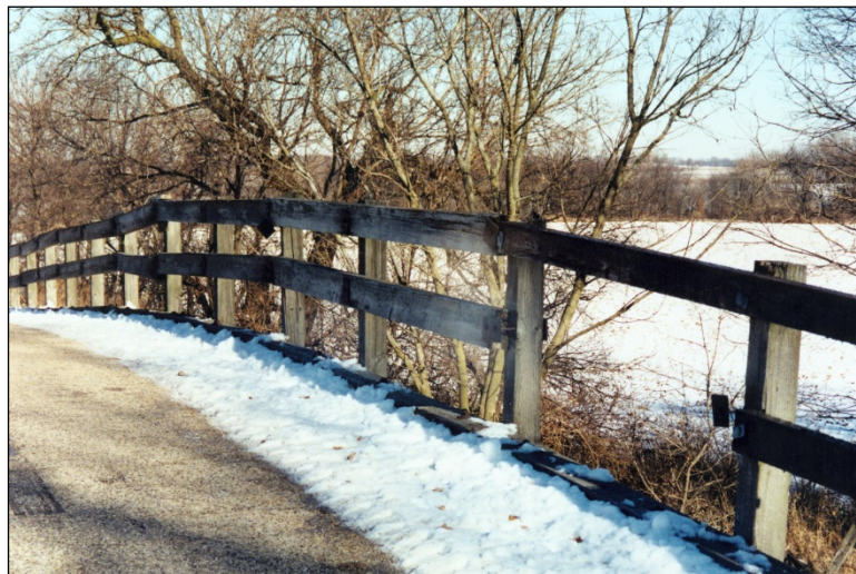
Figure 2.6.7.3-3 Missing Timber Bridge Rail Beam – Condition State 3
