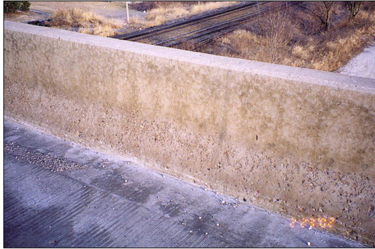
Figure 2.6.7.2-3 Scaling on the Lower Half of a Concrete Bridge Rail - Condition State 2
