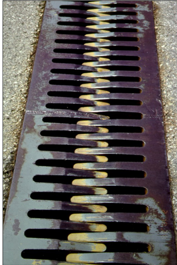
Figure 2.6.4.6-2: Finger Plate Expansion Joint – Condition State 1.
