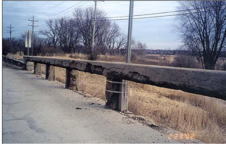
Figure 2.6.7.2-5 Concrete Bridge Railing - Condition State 4
