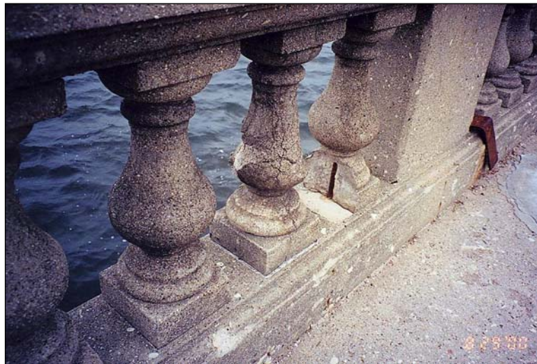
Figure 2.6.7.2-4 Ornamental Concrete Bridge Rail – Condition State 3
