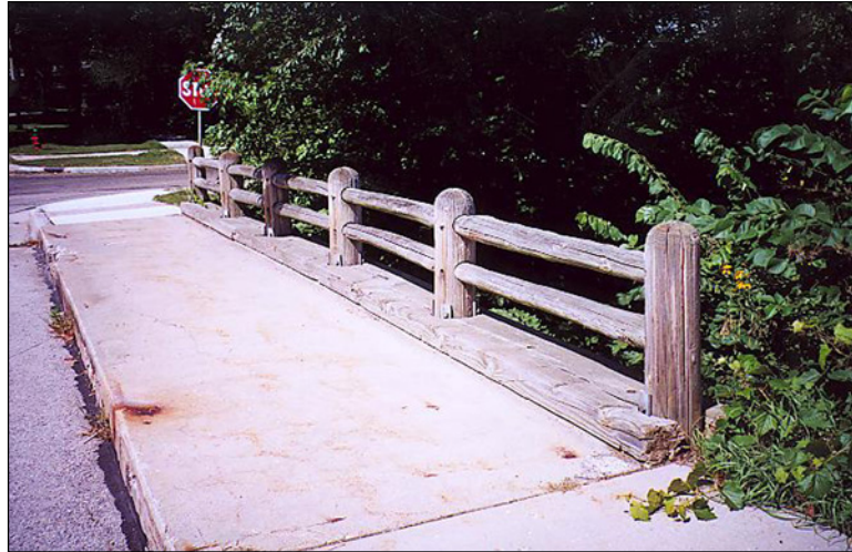
Figure 2.6.7.3-2 Timber Bridge Railing – Condition State 2
