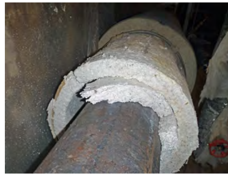
Asbestos wrapped utility pipes.
