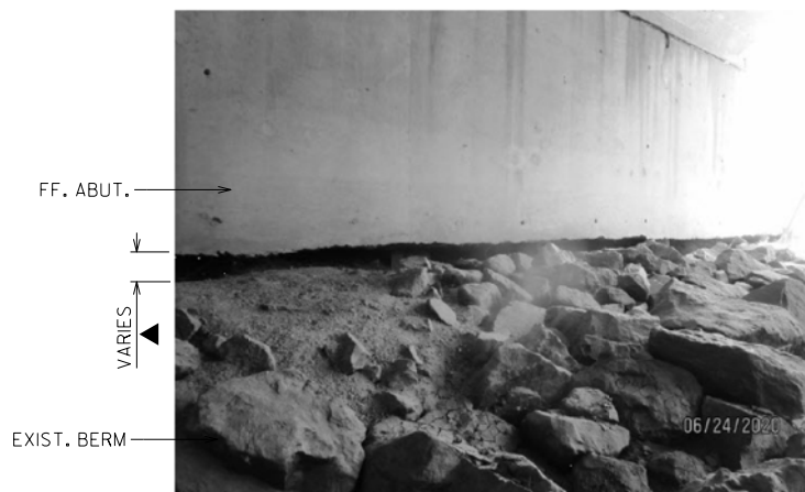
UNDERMINING AT B-11-137 N. ABUT.
