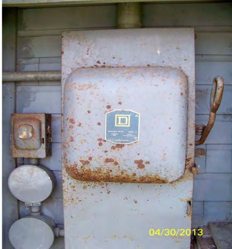
Machine/Storage Building Mechanicals
