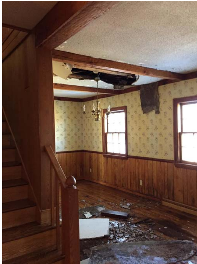
Water Damage from Upstairs
