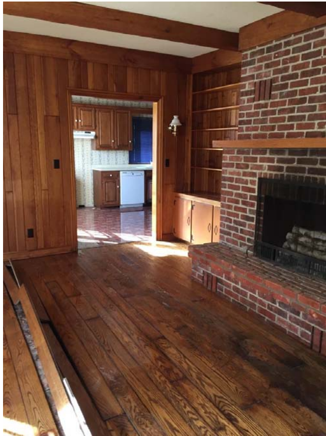
Living Room (Water Damage)
