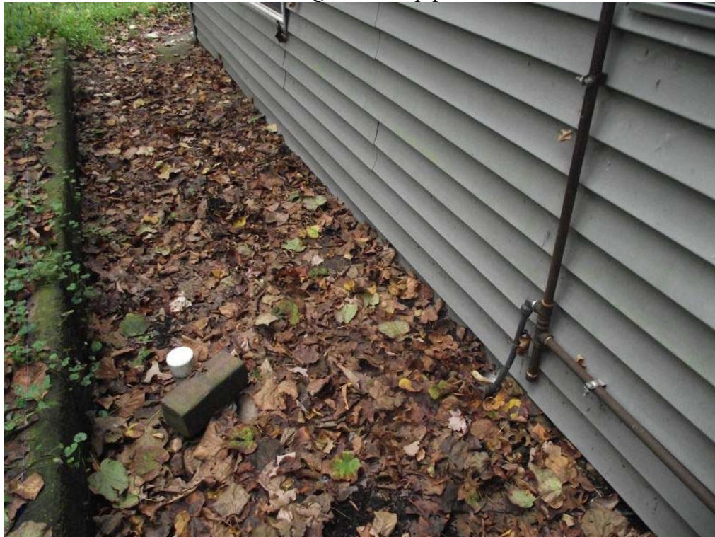
Gas connection at house near underground a/c pipes – concrete curb east of house
