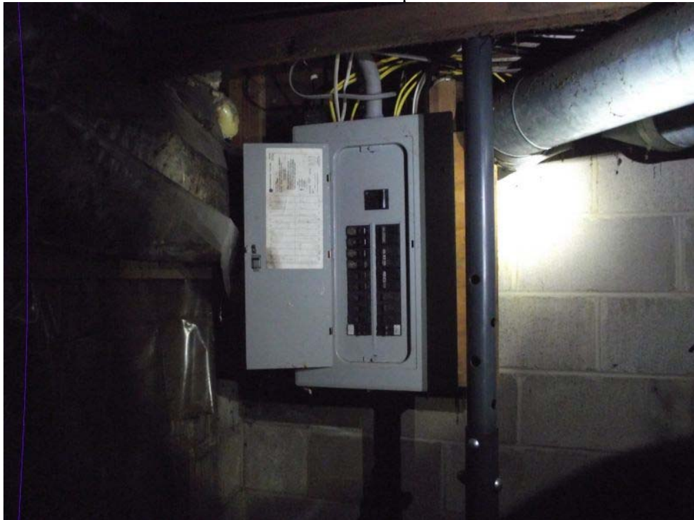
Electrical circuit panel
