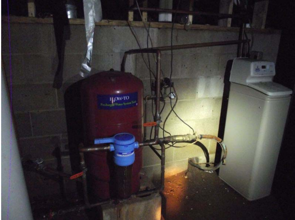
Water pump & softener in basement
