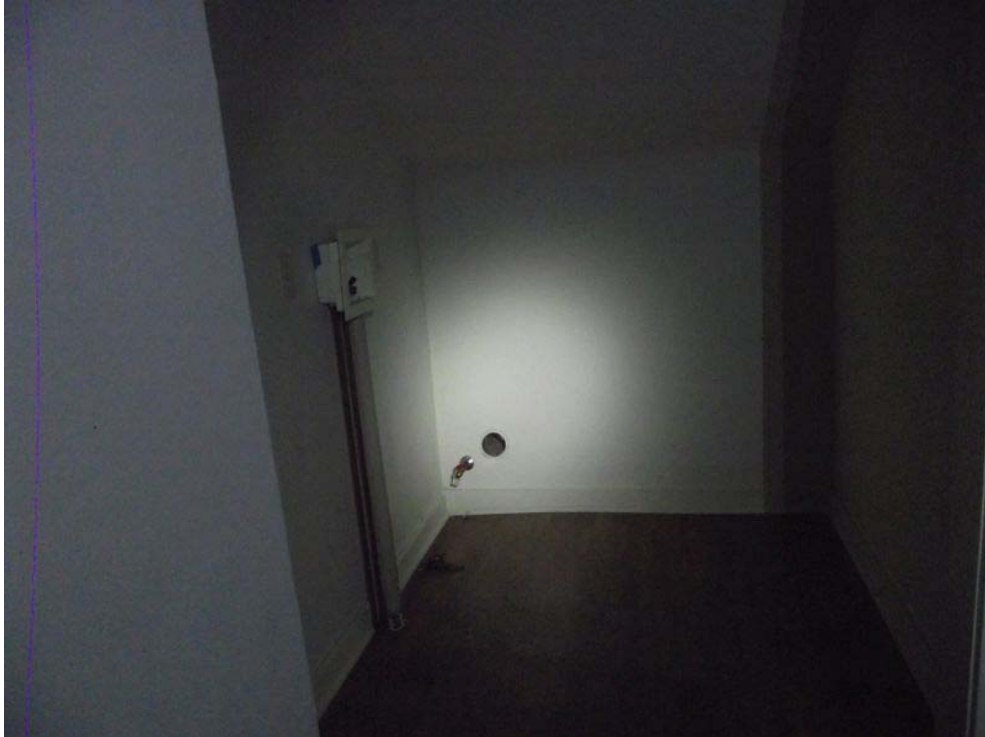
Washer hookup – gas line to dryer
