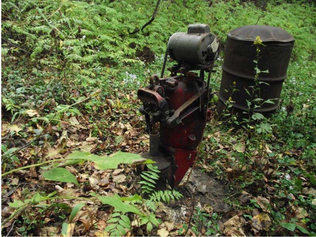
Well & motor under 55-gal drum
