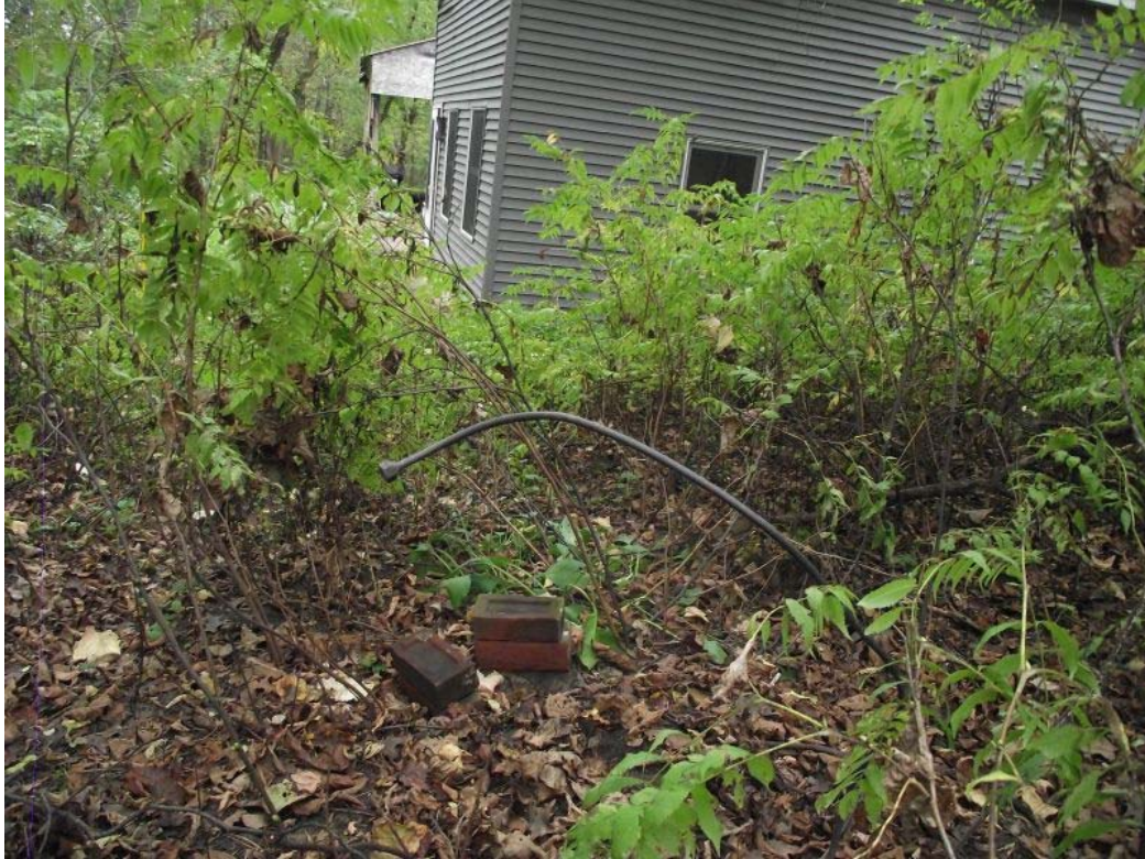
Gas line disconnected from LP tank – east of house
