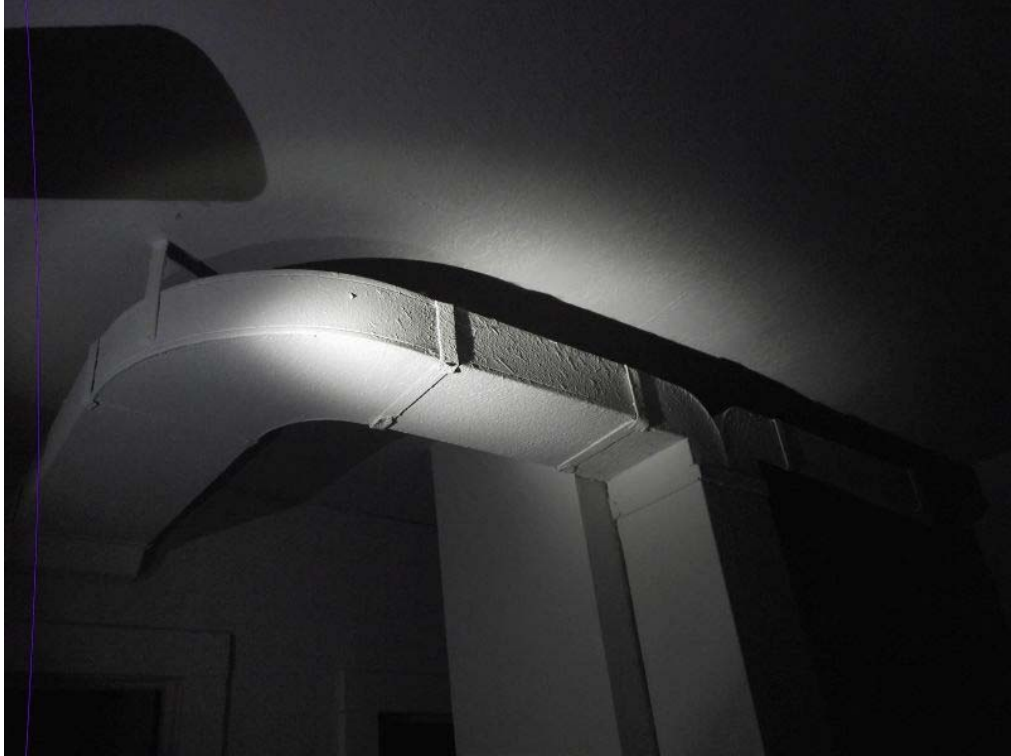
Upstairs duct work in hall
